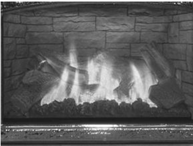
Photo 10 – Typical Burner Flame Appearance
