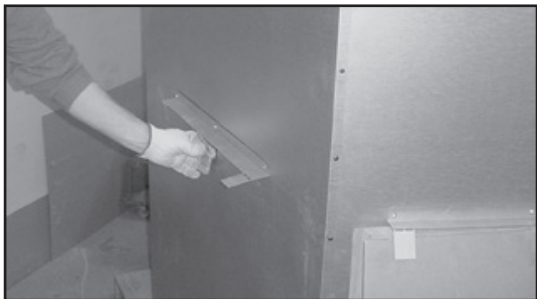
Figure 3.7 Bend Refractory Brackets Back Down
