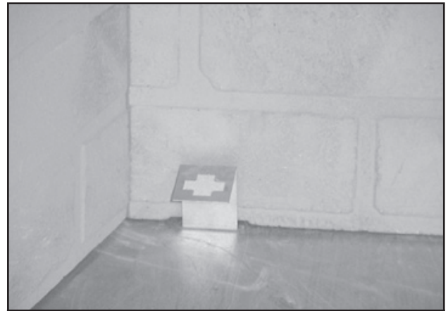
Figure 8.8 Grate Retaining Bracket in Place
