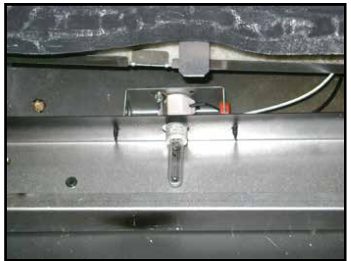
Figure 11.10 Ember Light Bulb Installed
