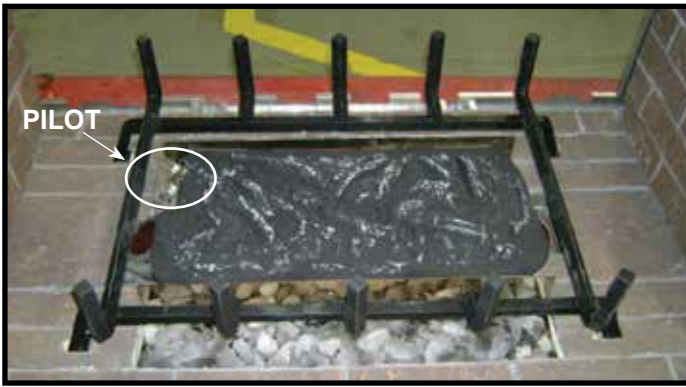
Figure 2. Burner and grate from front.
