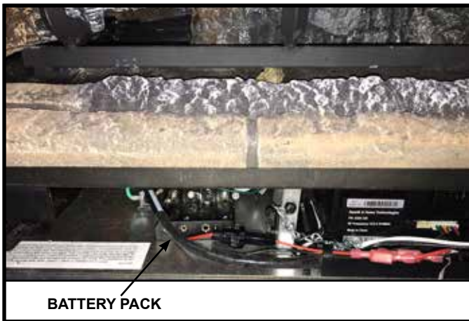
Figure 6.3 Battery Pack Installed
